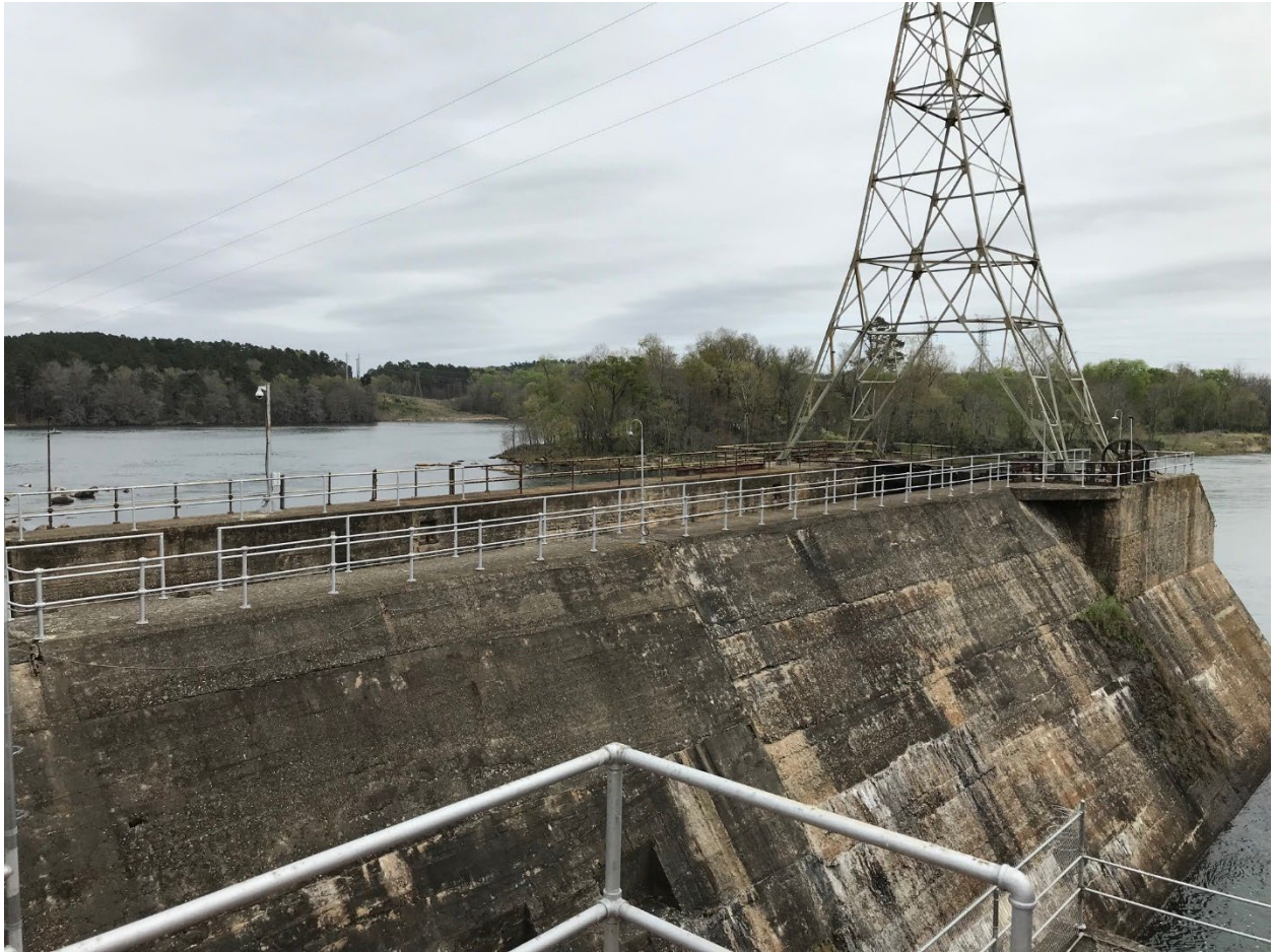
FIGURE 4.18 STEVENS CREEK PROJECT NAVIGATION LOCK, VIEW LOOKING DOWNSTREAM
