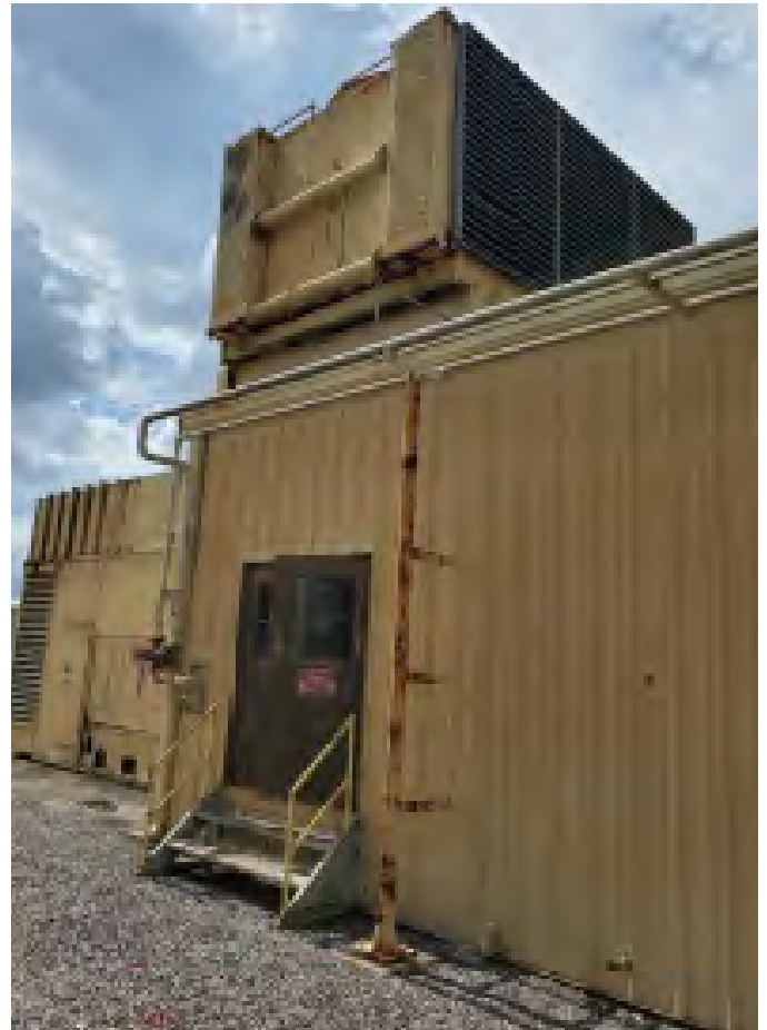
Bushy Park Combustion Turbine
