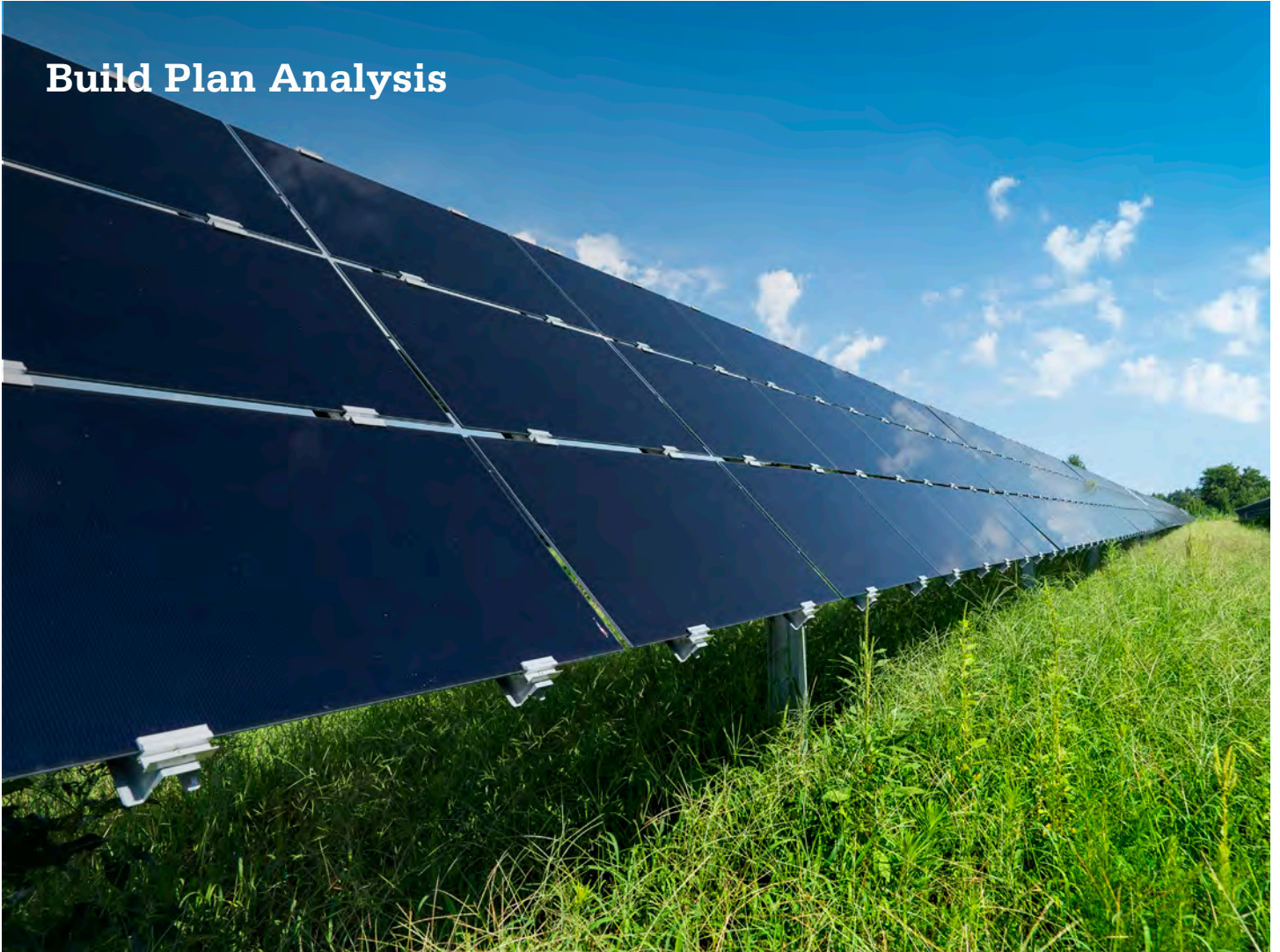
Springfield Solar Facility; Orangeburg, South Carolina
